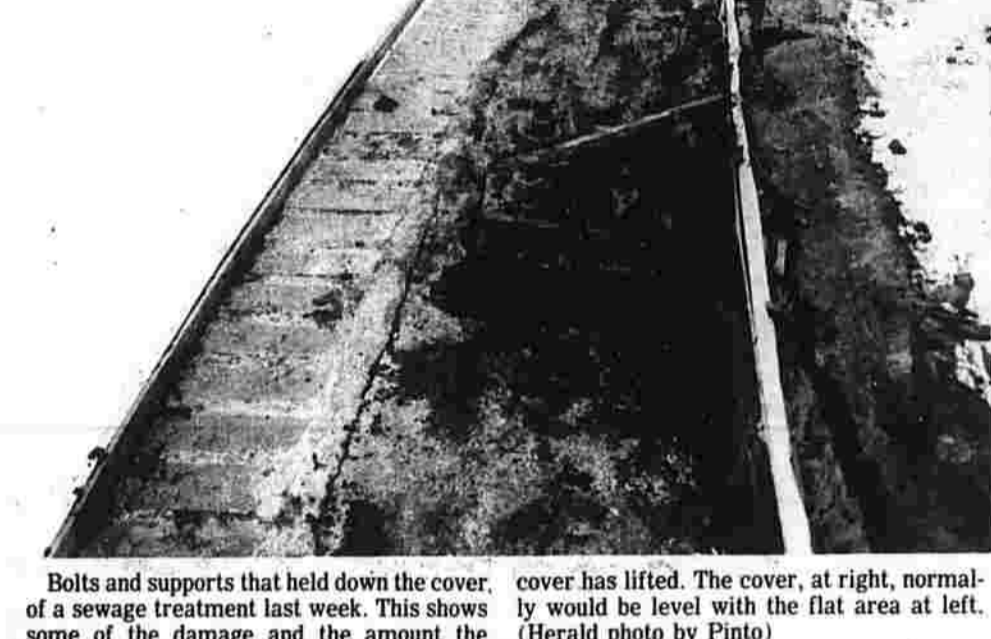
Bolts and supports that held down the cover, of a sewage treatment tank, were shown in this photo. The cover has lifted. The cover, at right, normally would be level with the flat area at left. Some of the damage and the amount the cover has lifted. (Herald photo by Pinto)
